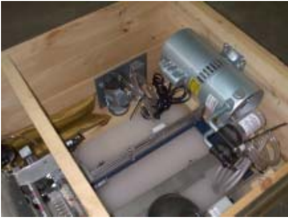
Air compressor is also secured to side of crate. Notice the wood brace across the middle of the crate
